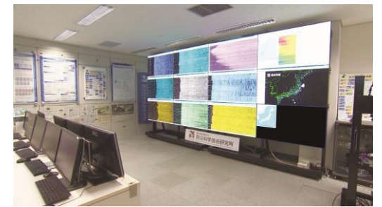
NIED's earthquake, tsunami, and volcano monitor room
